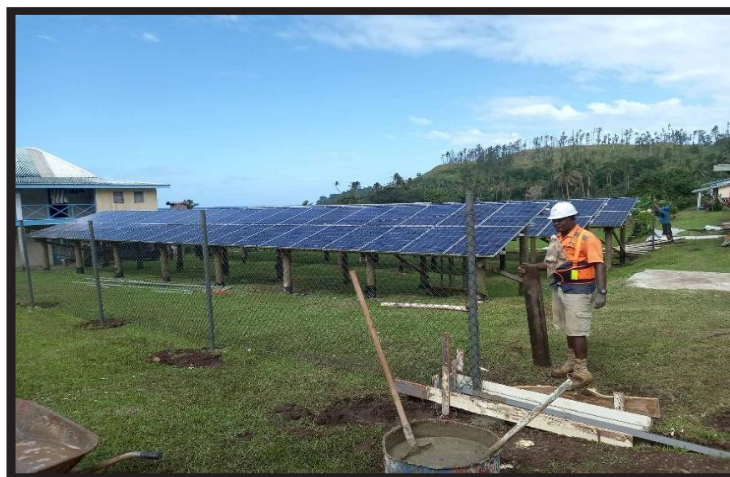
Figure 4: Solevu Solar Hybrid Project
